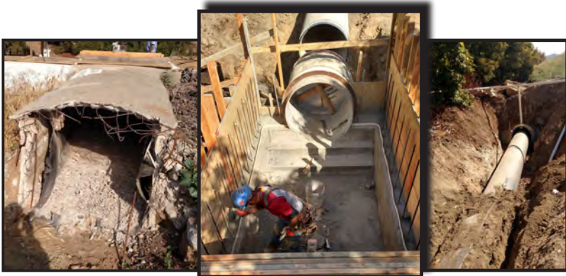
Cover pictures: Vista Flume Relocation Project. Description of the project is available on page 11.
