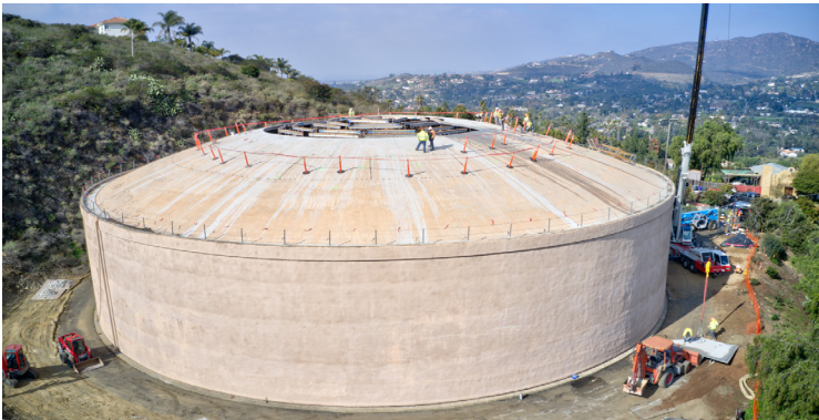
Cover photos: Top: Buena Creek (HB) Reservoir circa 1960's Bottom: Buena Creek (HB) Reservoir rehabilitation in progress
