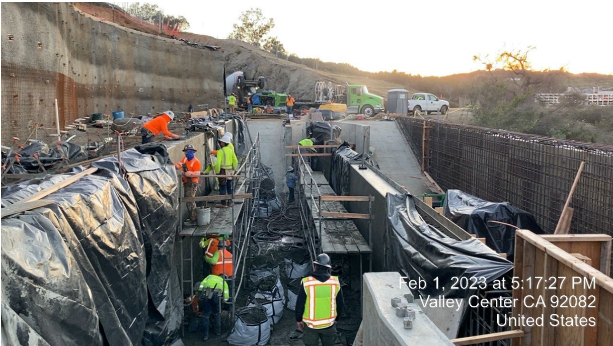
Crew finishing the shotcrete installed to provide smooth surface. All work is inspected for conformance
