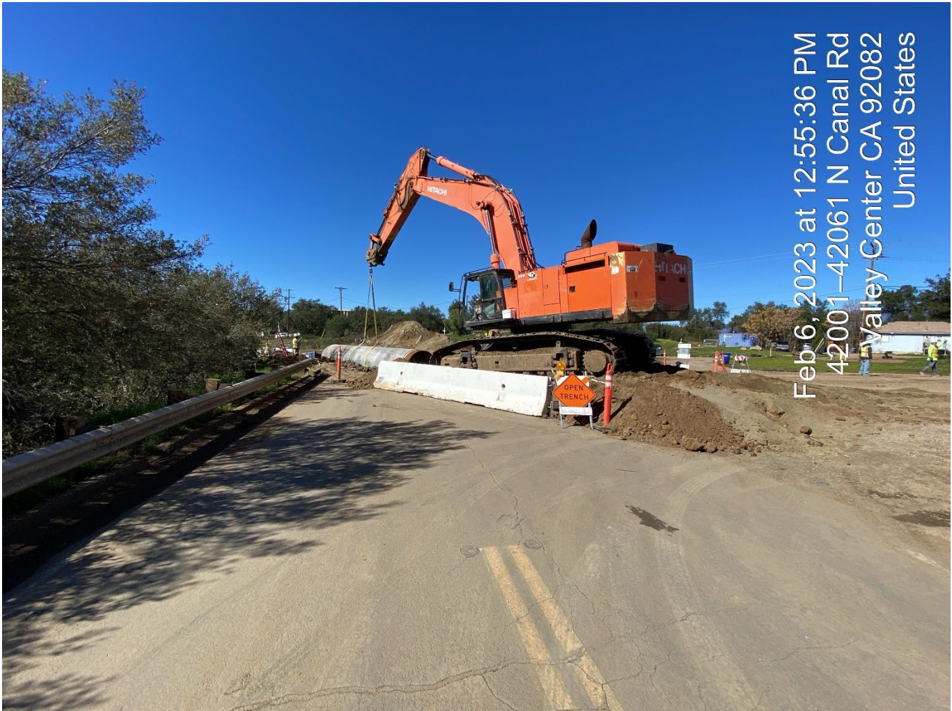
Canal road closure for installation of the CMLC pipe within the intersection of Tokama and Canal Rd.
