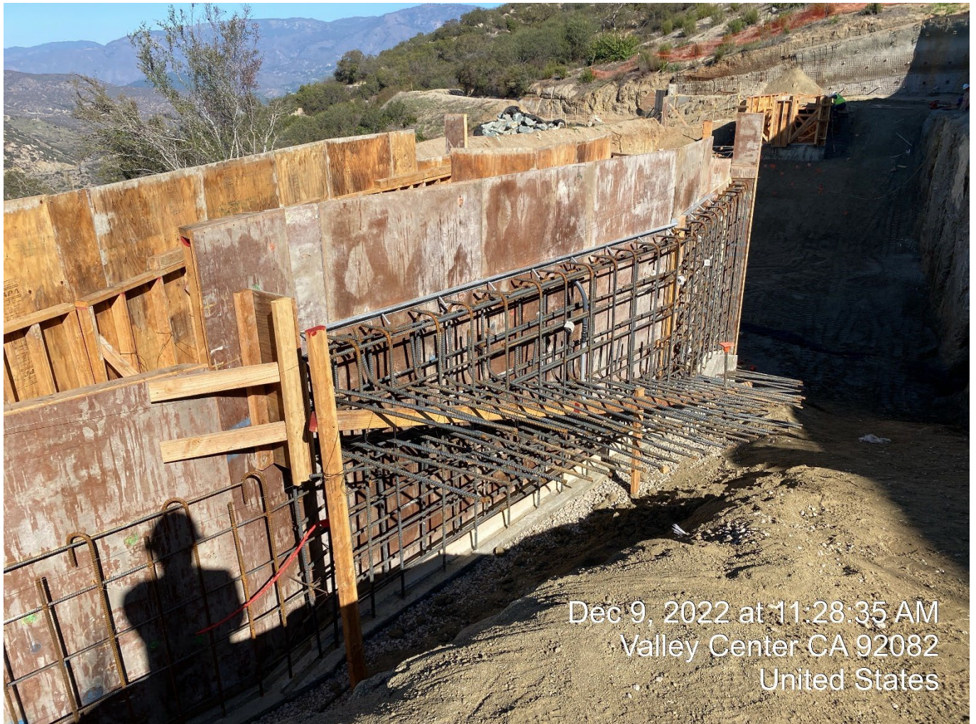
Rebars and forms for the inlet / outlet walls for the desilting basin were installed and inspected
