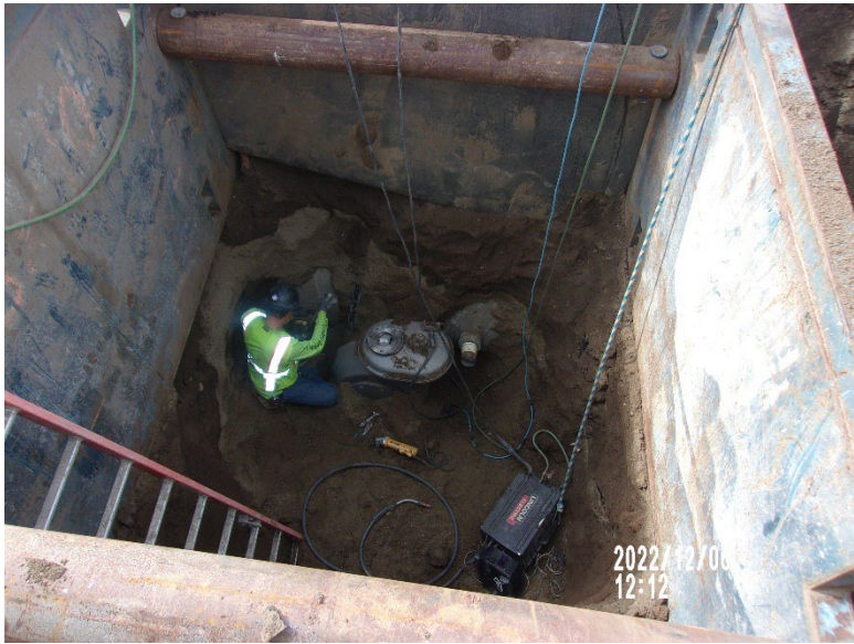
Bypass pipe as part of the pump-out structure
