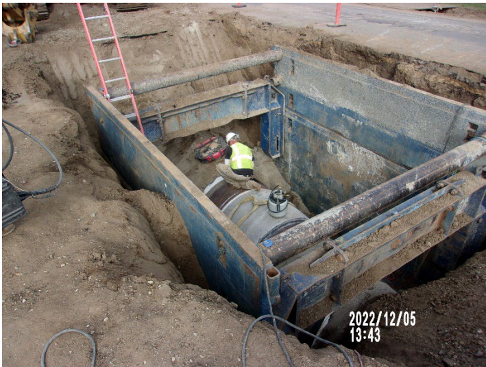
Crew connected the north end of the pump out structure to the 60" CMLC pipe that was installed earlier. The outside joints as well as the interior joints were welded.
