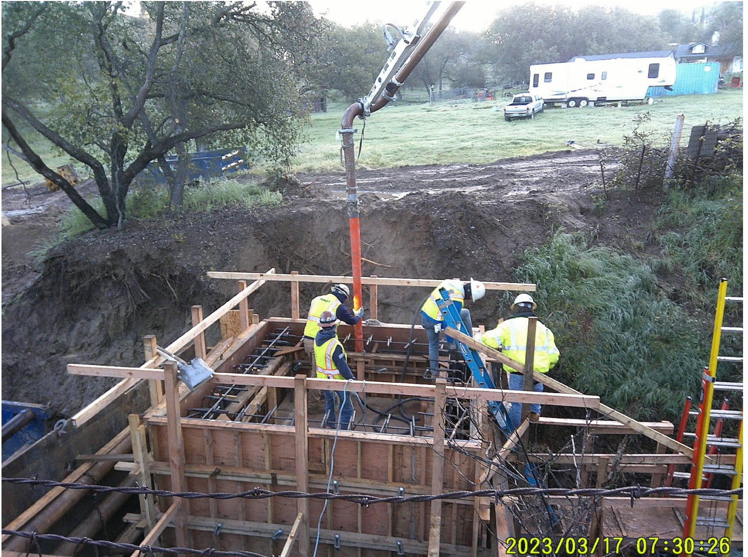
Placing concrete for the S. terminal structure wall. The top of the structure will be poured this week
