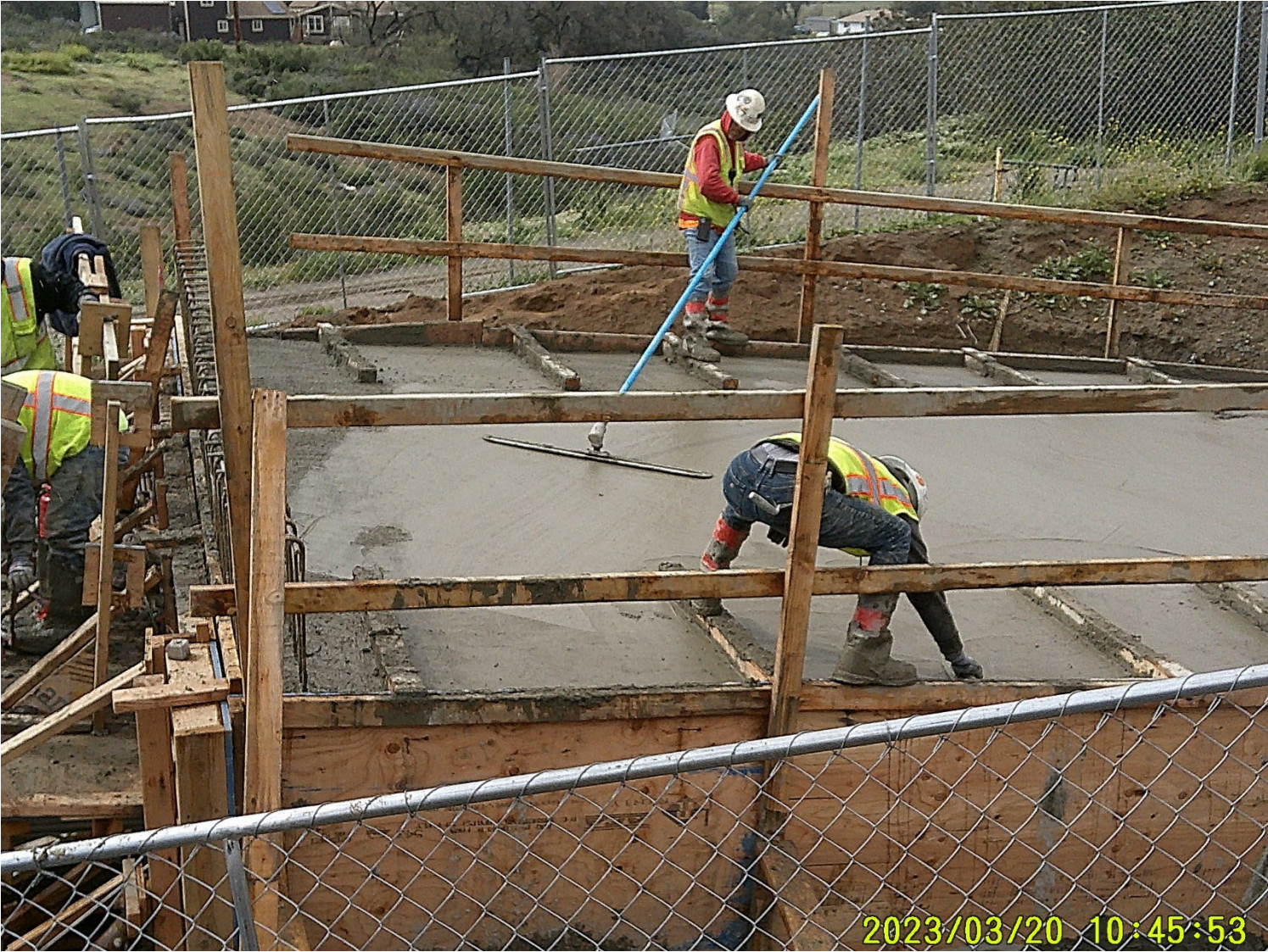
500 yards of concrete poured for the second half of the access tunnel started at 4:00 am. on Monday 3/20
