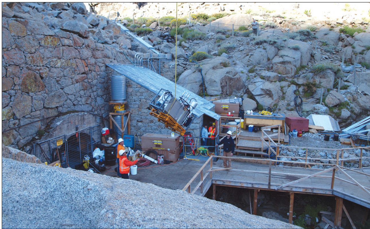
The recent project for Pacific Gas and Electric in the Sierra Madre mountains was unique, because this very old natural rock dam structure was in need of rehabilitation and was located in a remote area accessible only by helicopter and pack animals.
