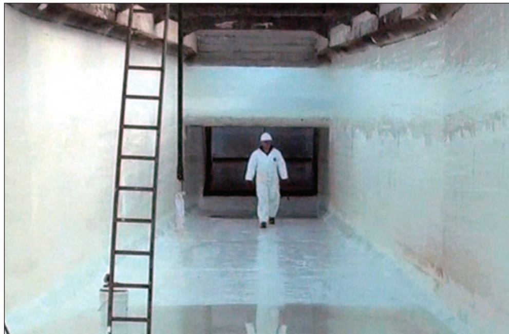
The Liawenee Flume located in Tasmania, was in need of structural rehabilitation with a material approved for drinking water use, after it was treated with Warrens' single-coat, high-build properties, structural values and zero volatile organic compound formulation.
