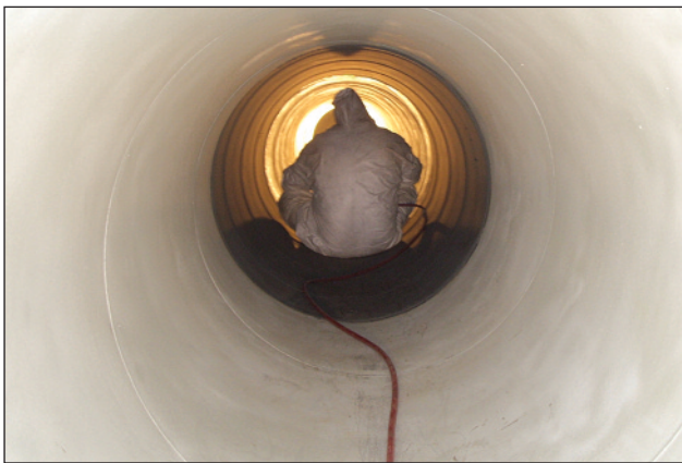
A man working in a pipe, one of the many jobs for which Warrens' products that are non-hazardous, and are safe to use in confined space are in such great demand.
