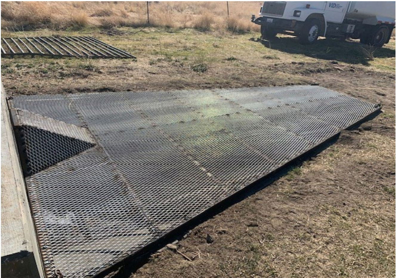
Improved Cover Eliminates Fall Hazard
