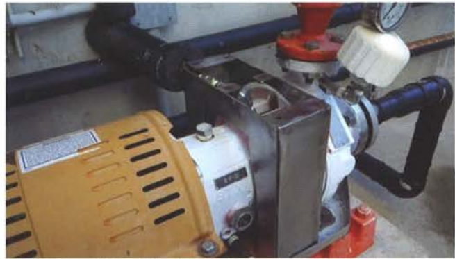
Central Coast Water Authority – Maintenance staff at the water treatment plant fabricated a splash shield to prevent contact with caustic soda solution during a seal flush of the suction pump.
